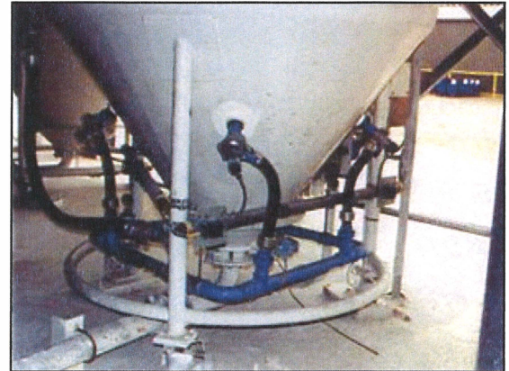
VA-12 AirSweep System mounted to the bottom of TiO 2 hopper.
